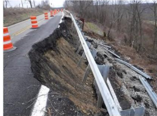
Photo 4: Photo looking South on SR 376 at landslide area on West side of SR 376
